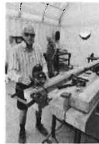
Shedder Michael Galloway working on the pergola uprights which will have the six panels inset into them.
