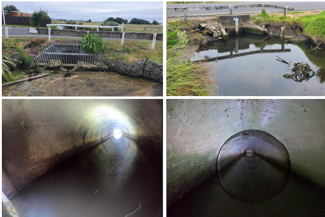
Figure 2-3 : Site Visit Photographs (12/10/2022). Top left: Inlet; Top right: Outlet; Bottom left: pipe interior; Bottom right: pipe interior
