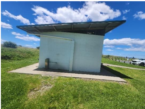
Push button shower – Roadside of the toilet block. $1,500 +GST
